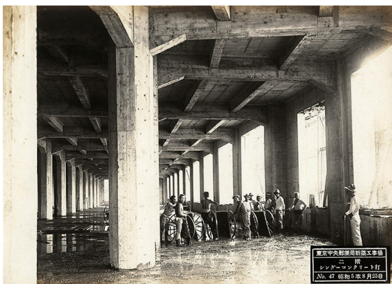
Construction Site of the New Tokyo Central Post Office, "Second-floor Cinder Concrete Pour", No. 31, August 25, 1930
